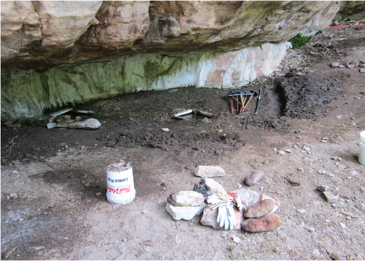
Fig. 6.11: Before restoration of the site, there were several very small catchments. Seepage emerged from the bedrock walls of coconino sandstone. Species were unable to establish themselves.
