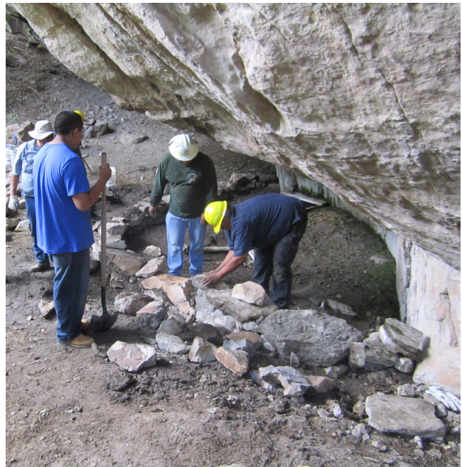
Fig. 6.10: Tribal partners helped to remove old corral fencing that was no longer functional.
