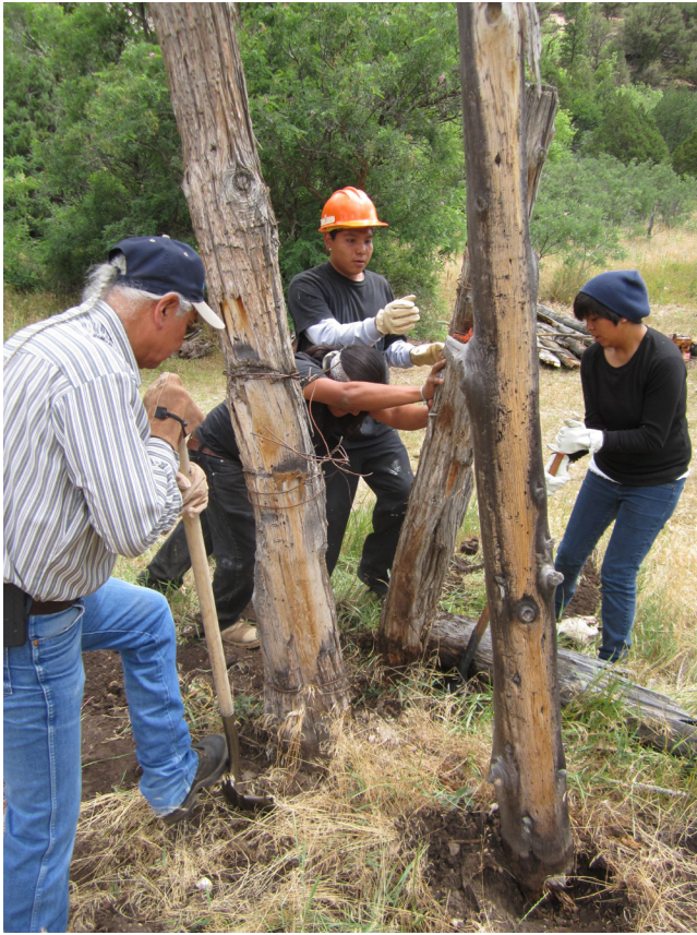
Fig. 6.08: Tribal partners helped to remove old corral fencing that was no longer functional.
