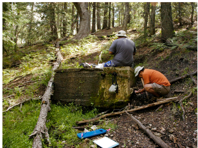
Fig 1.13: This spring was excavated and boxed long ago. The piping is no longer functional, so the flow pours out onto the ground.
