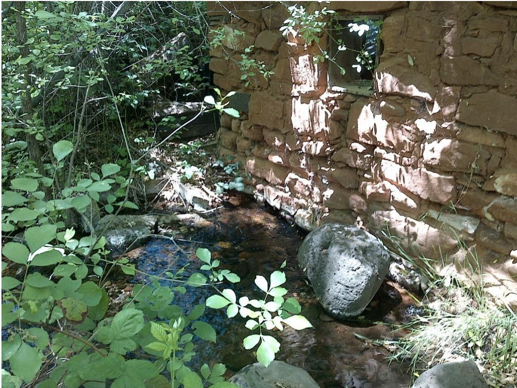
Fig 30.1 Thompson Springhouse Spring: Flow emerges from the downstream (southeast) side of the historic springhouse, forming a springbrook.
